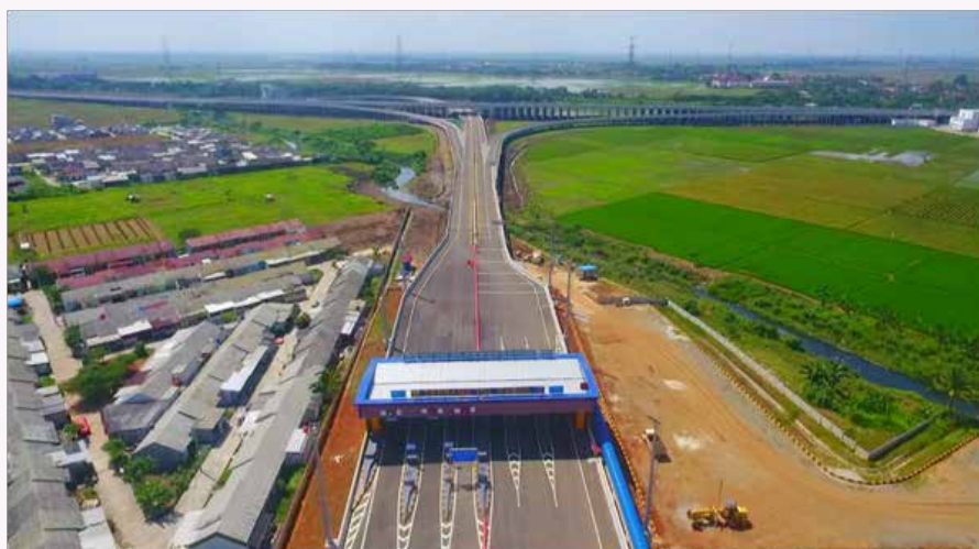
Gambar Progres Seksi II Jalan Tol Cibitung Cilincing Progress of Section II of the Cibitung-Cilincing Toll Road
