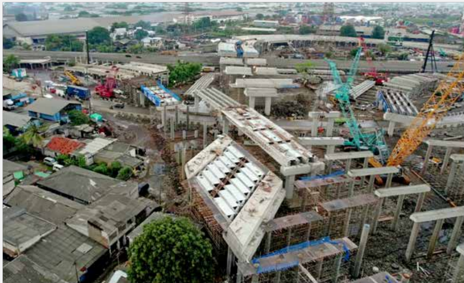
Gambar Progres Seksi IV Jalan Tol Cibitung Cilincing Progress of Section IV of the Cibitung-Cilincing Toll Road
