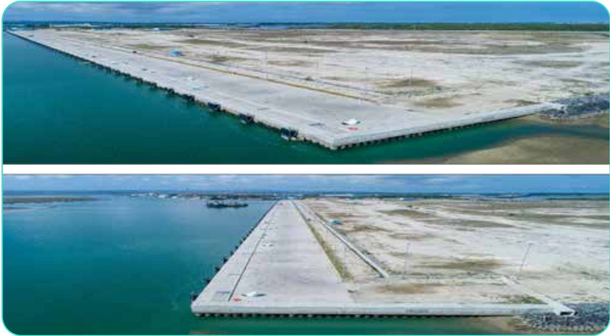
Gambar Dokumentasi Pekerjaan Revetment dan Retaining Wall Dumping 2 dan Dermaga Curah Cair Revetment Work Documentation and Retaining Wall Dumping 2 and Liquid Bulk Jetty
