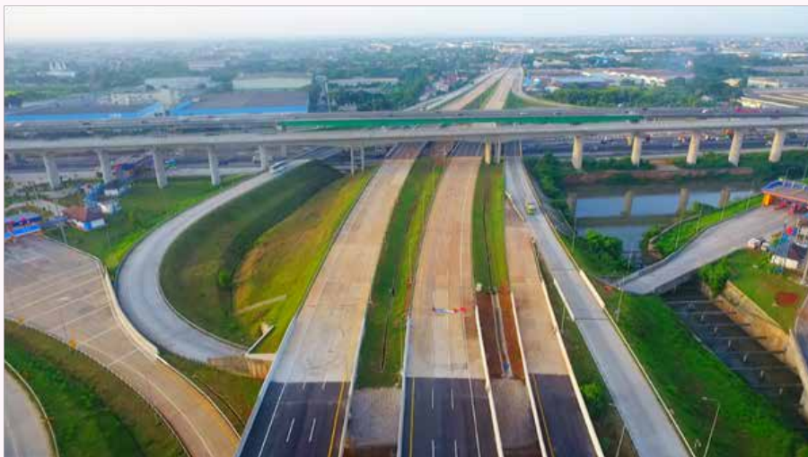
Gambar Progres Seksi I Jalan Tol Cibitung Cilincing Progress of Section I of the Cibitung-Cilincing Toll Road
