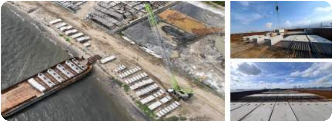
Gambar Area Stockyard Precast Tie Beam dan Pile Cap Stockyard Area Precast Tie Beam and Pile Cap
